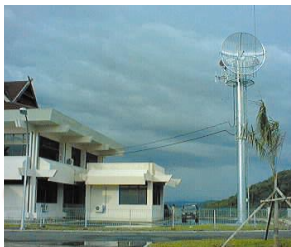
Bili Bili Dam Telemetry System (Indonesia)
