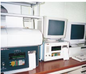
Nikko Sabo Dam Supervising and Information System (Japan)
