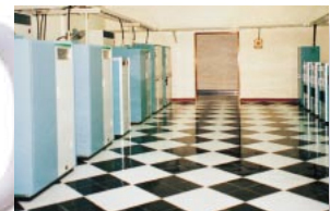
Vietnam Coastal Communication System Hai phong- Transmitting
