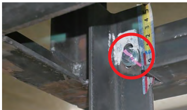
図9 ストラクチャ代替架台と振れ止め金具の接合部 Fig.9 Joint between structure alternative frame and anti-sway bracket
