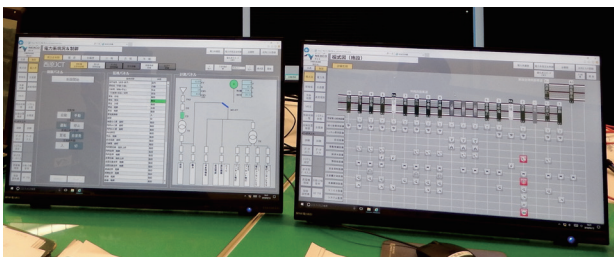
図6 操作卓 Fig.6 Control Terminal
