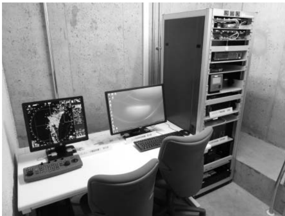
図3 屋内機器 (センサ側) Fig.3 Indoor Equipment (Sensor Station)
